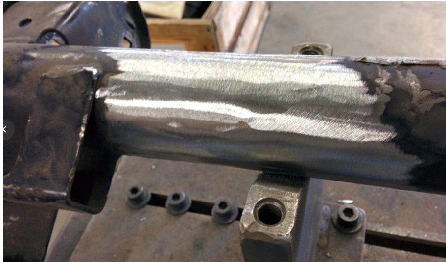
Figure 2. Upper Control Arm Bracket Removed and Cleaned Up
